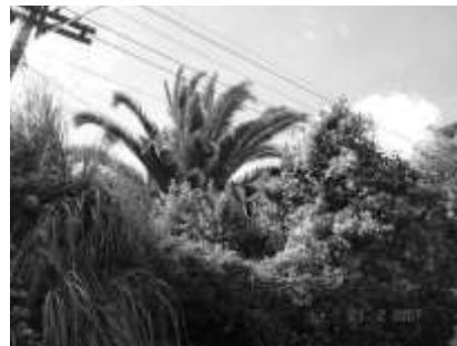
Trees close to powerlines Feb 2007
