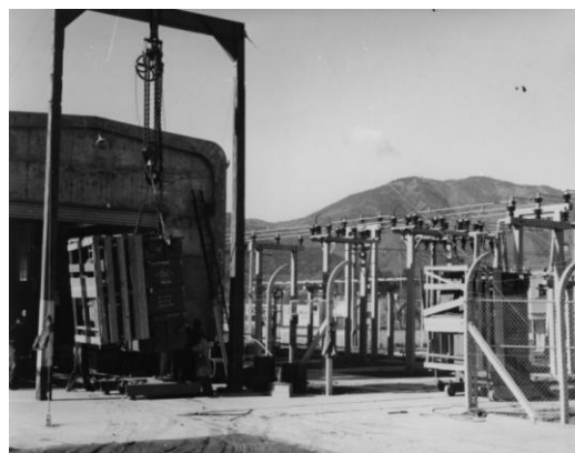
NEL's 33kV transformers arriving in Jan 1960
